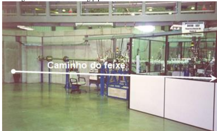
Figure 3: Photo of the ring pipe for the DO9B – XRF line of LNLS.
