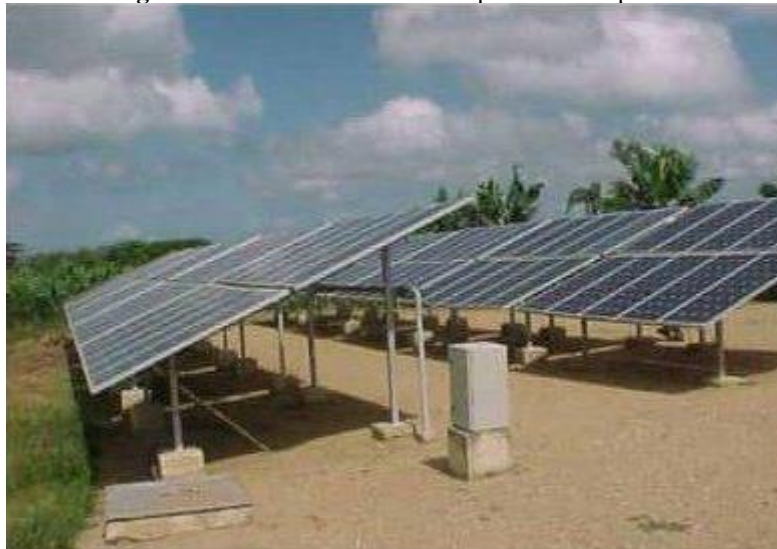
Figure 2. Santa María del Lotero photovoltaic plant.
