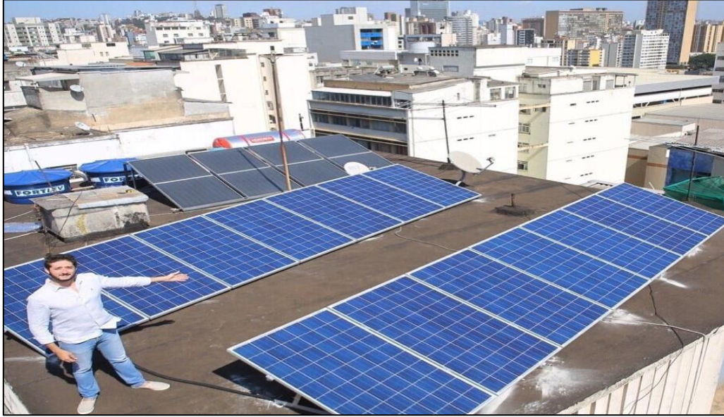
Figure 4. Installation of modules with the inclination for bifacial panels on concrete roof
