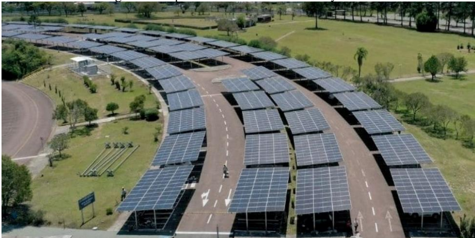
Mini generation plant at the Federal University of Paraná.
