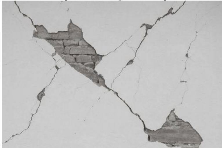
Figure 12 – Masonry with cracking.
