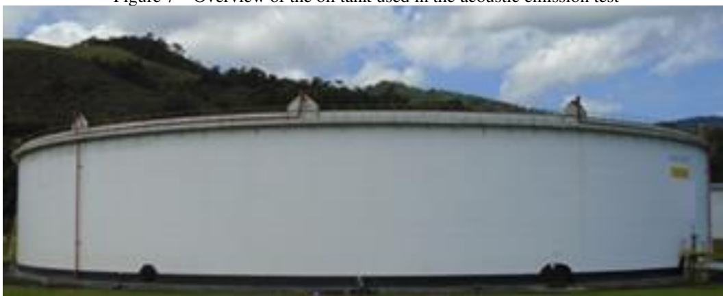
Figure 7 – Overview of the oil tank used in the acoustic emission test
