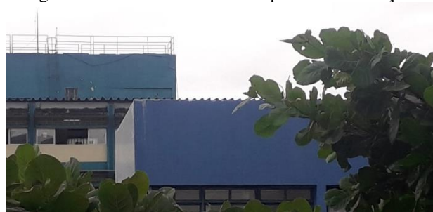
Figure 2 - Efflorescence at the top of the front façade
