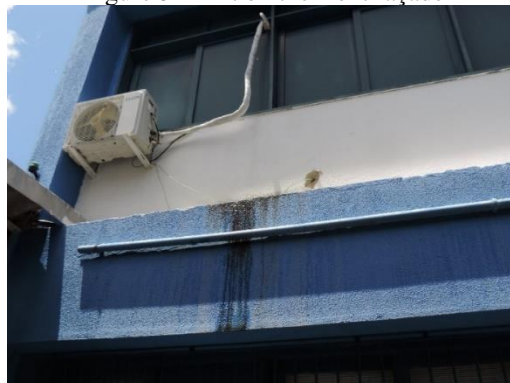
Figure 3 - Dirt on the front façade
