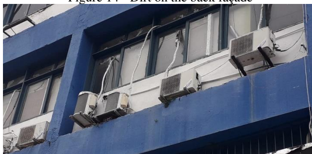
Figure 14 - Dirt on the back façade
