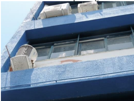
Figure 5 - Detachment of the painting near the windows
