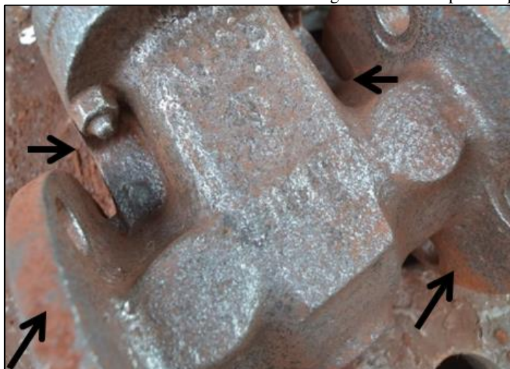
Figure 7: Treatment with Needle Gun still showing corrosion and paint deposits.
