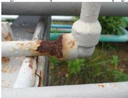
Figure 1: Atmospheric Corrosion in Piping.
